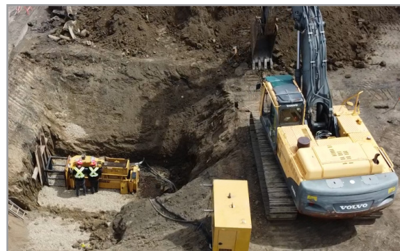
Figure 3. Aerial View of Static Pipe Bursting Machine and Machine Pit – 62 nd Avenue
