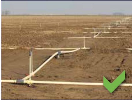
Certa-Set pipe entirely installed in an "H" design pattern
