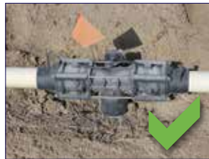
Nelson valve with burried mainline
