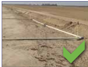
Swing joints are on both sides of the Nelson valve
