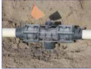
Nelson valve with buried mainline
