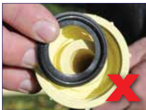
Incorrect O-ring positioning
