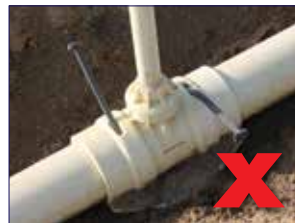
Spline not inserted in same direction
