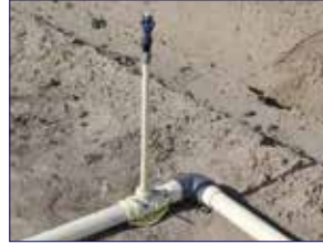
Elbows connecting lateral pipe runs
