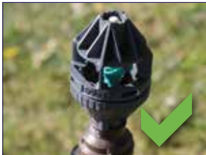
Sprinkler head installed
