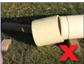
Misaligned pipe and coupling
