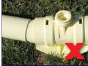
Misaligned pipe and sled coupling
