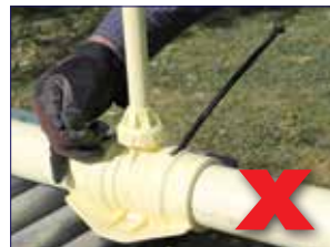
Spline not fully inserted
